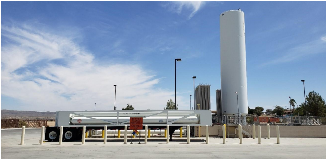
Figure 8-9. Barstow Yard Existing CNG Facilities
