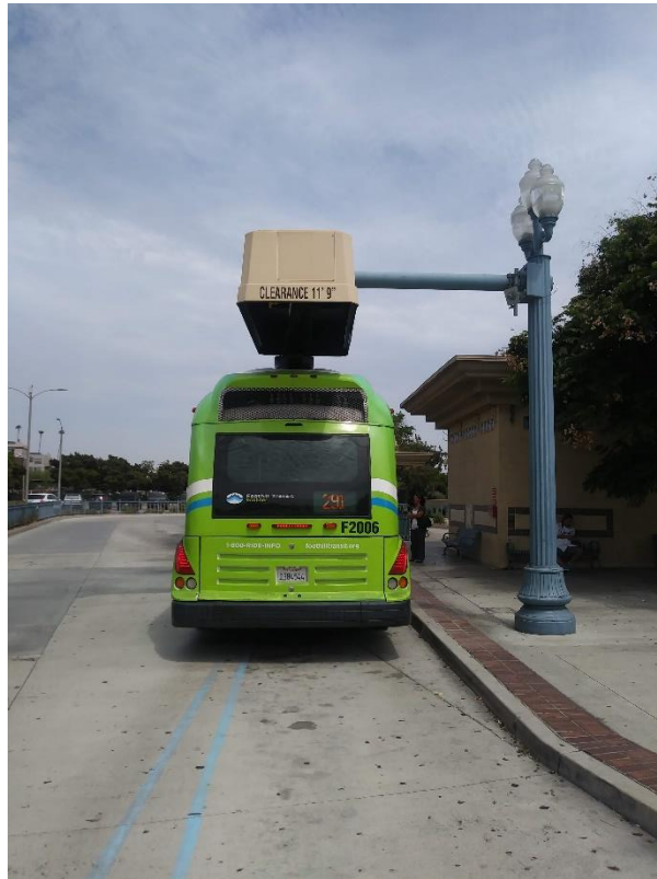
Figure 1-13: Pomona Transit Center On-Route Charger Multifunctionality
