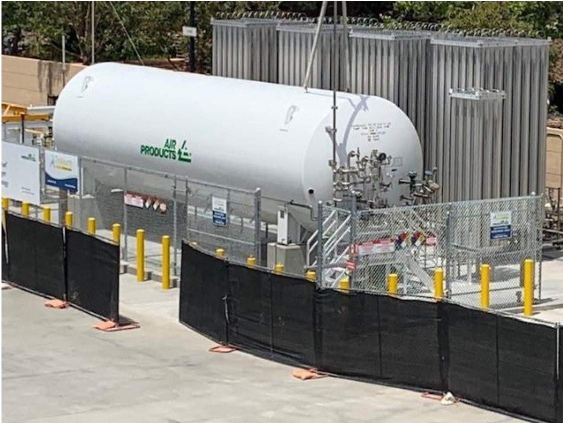
Figure 2-4. 4,500kg hydrogen tank located at Orange County Transit Authority (OCTA) designed to serve 50 FCEB buses.
