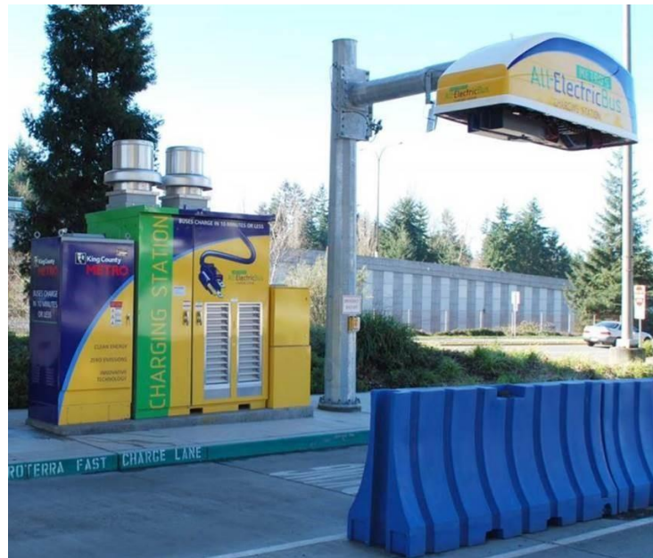
Figure 1-16: King County Metro Branded On Route Charger
