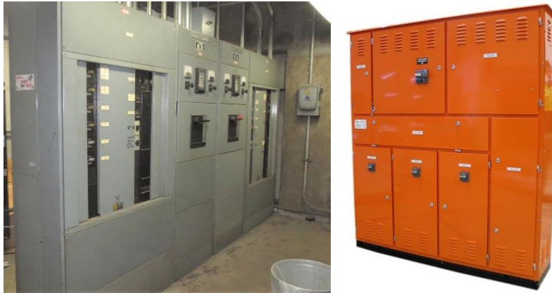
Figure 1-4: Interior and Exterior Switchboard
