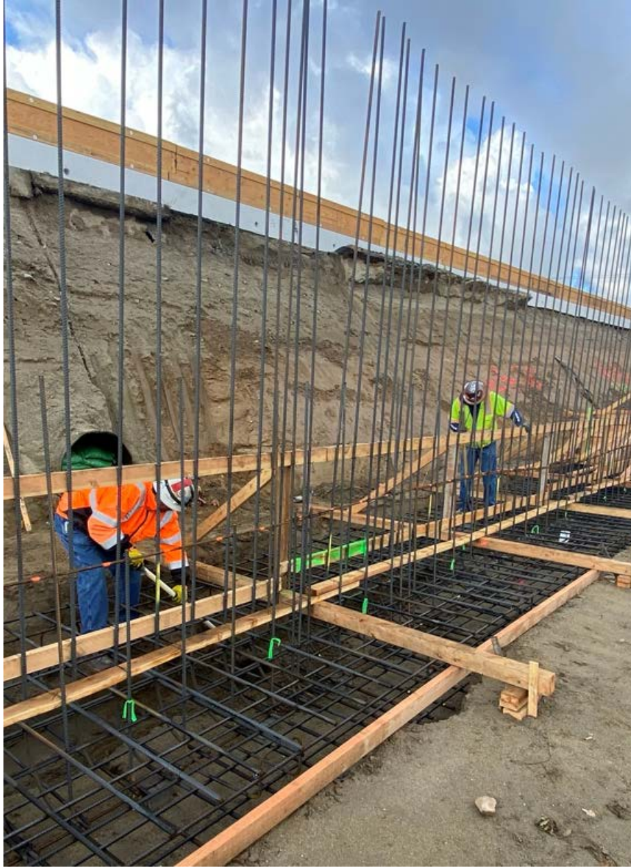
Helping to mitigate anticipated sound impacts is just one of the many features of the I-10 Express Lanes Project. Here, crews prepare the foundation of a sound wall in the western part of the county.
