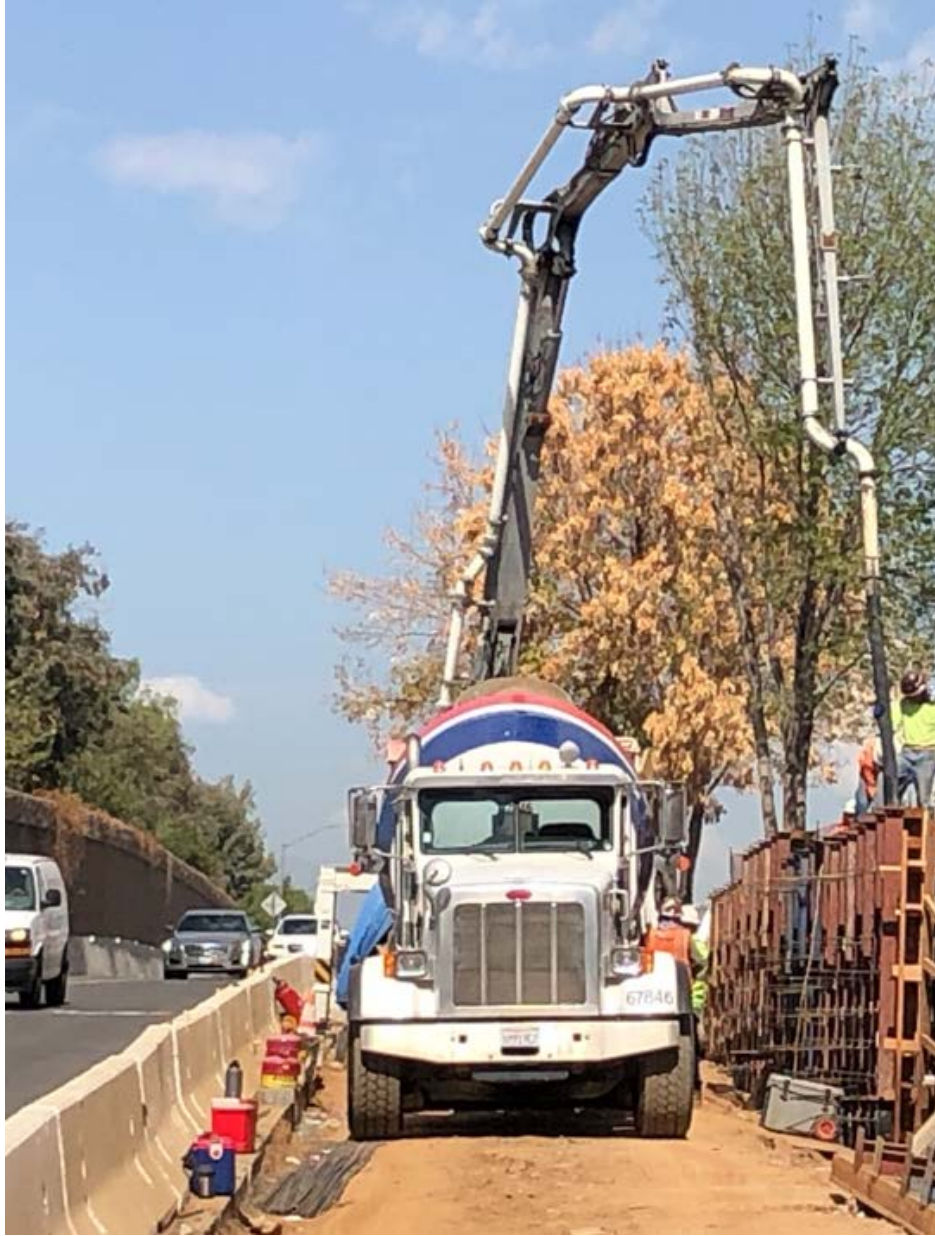
A pumper truck supplies the concrete used in the footings for new retaining walls at the Interstate 10 (I-10) University Interchange in Redlands.
