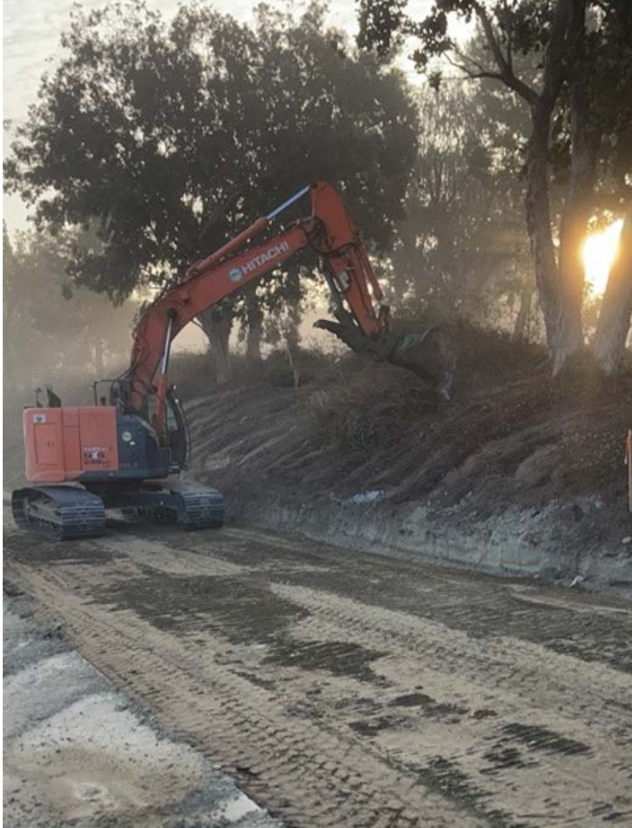
Early morning crews excavate a slope to allow for the widening of ramps at State Route 60 and Central Avenue in Chino.
