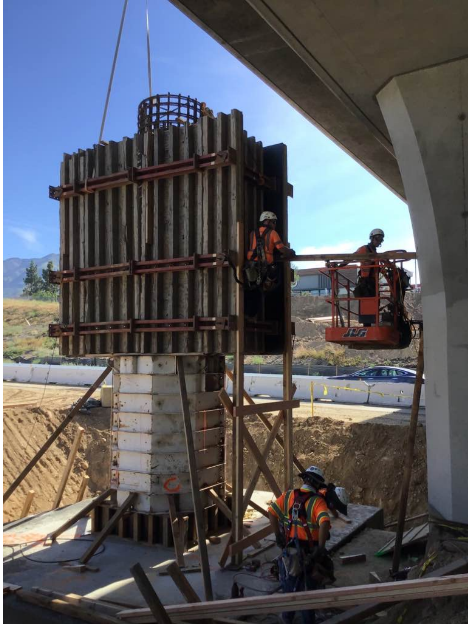
Large wooden forms are built to construct bridge columns at the Baseline Interchange on State Route 210 (SR 210) in Highland.
