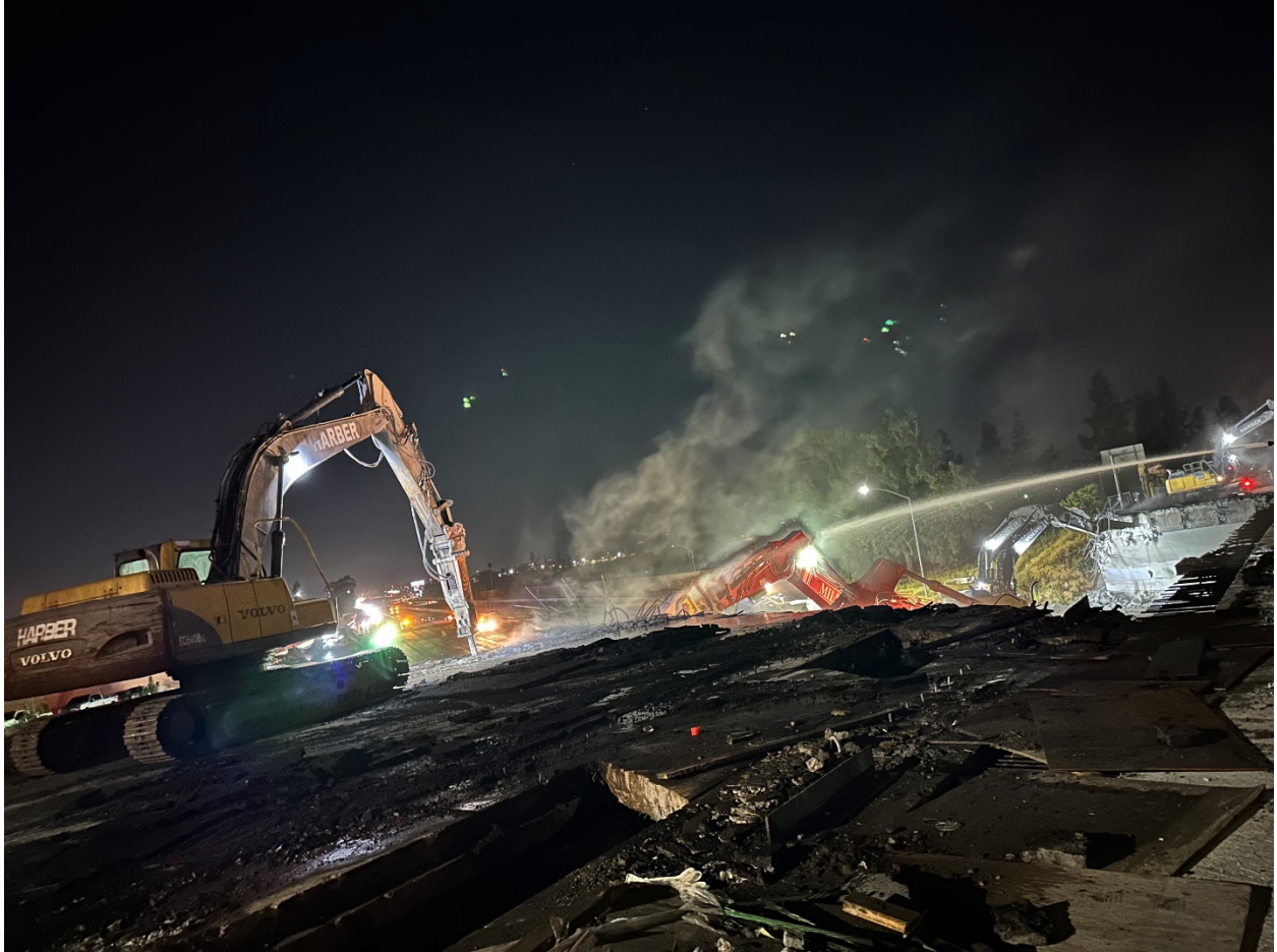
Nighttime work is necessary to minimize disruption to the traveling public. Crews are seen here demolishing the Vineyard Avenue bridge.
