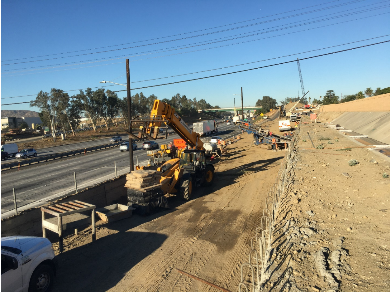
Preparing for the installation of new retaining walls along the ramps at Cedar Avenue in Bloomington, crews install the soil nail system for additional strength of the walls.
