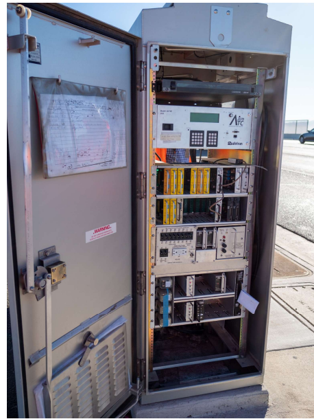
I-15 interchange southbound offramp traffic signal (TEES)
