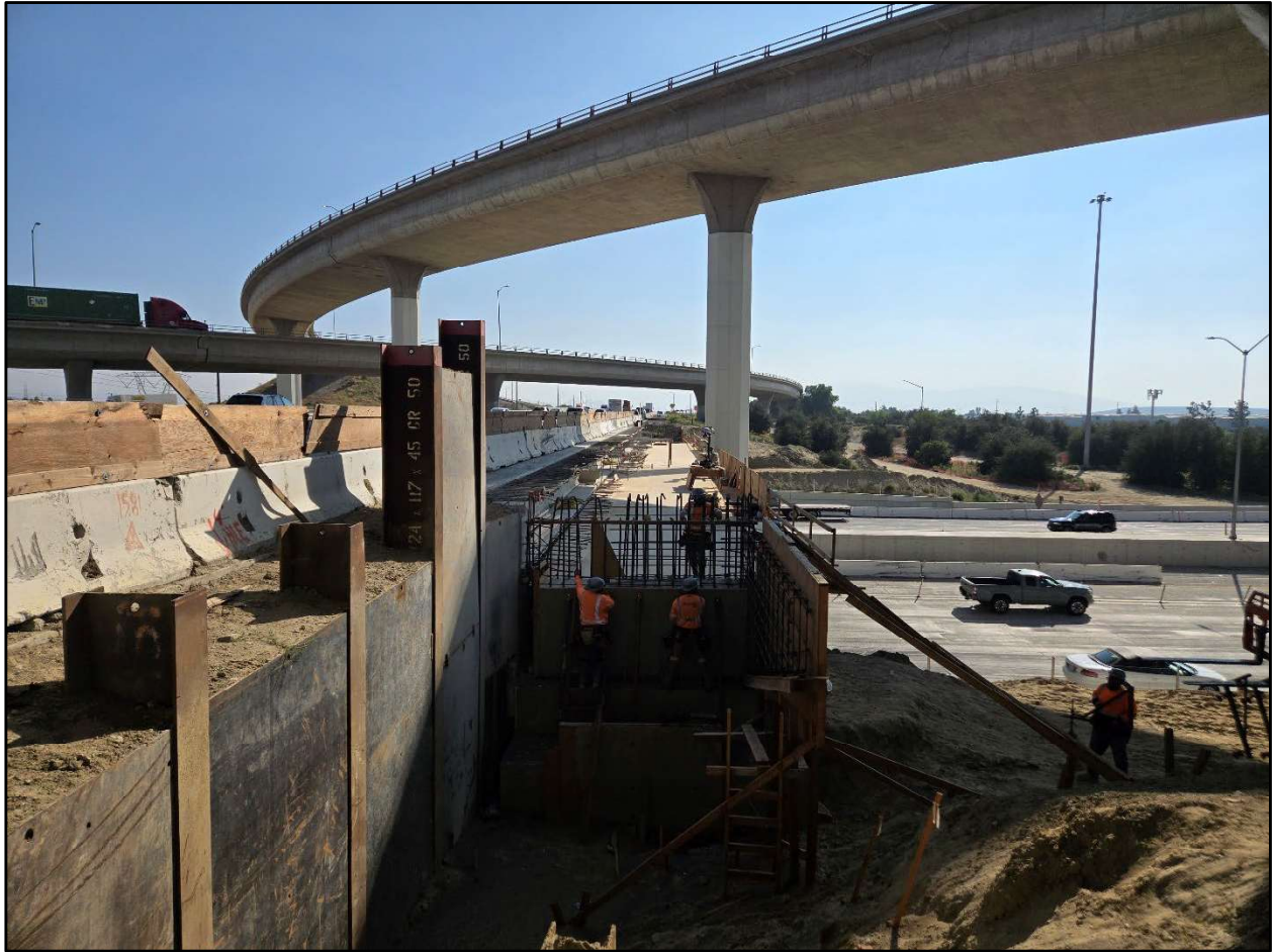
Interstate 15 (I-15) Corridor Freight and Express Lanes: Crews work on the I-15 Corridor, building the new, wider I-15 deck over the Interstate 10.
